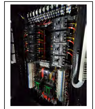
Power Cabinet Box
